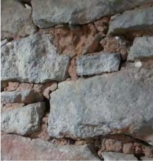
Fig. 5: Example of earth mortar, used as dug, from very close to site, Main St. Longforgan, early 19th C. Shrinkage cracks as a result of high clay content in chimney wall.
