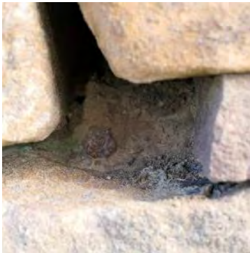
Fig. 18: Earth mortar, severe external decay.
