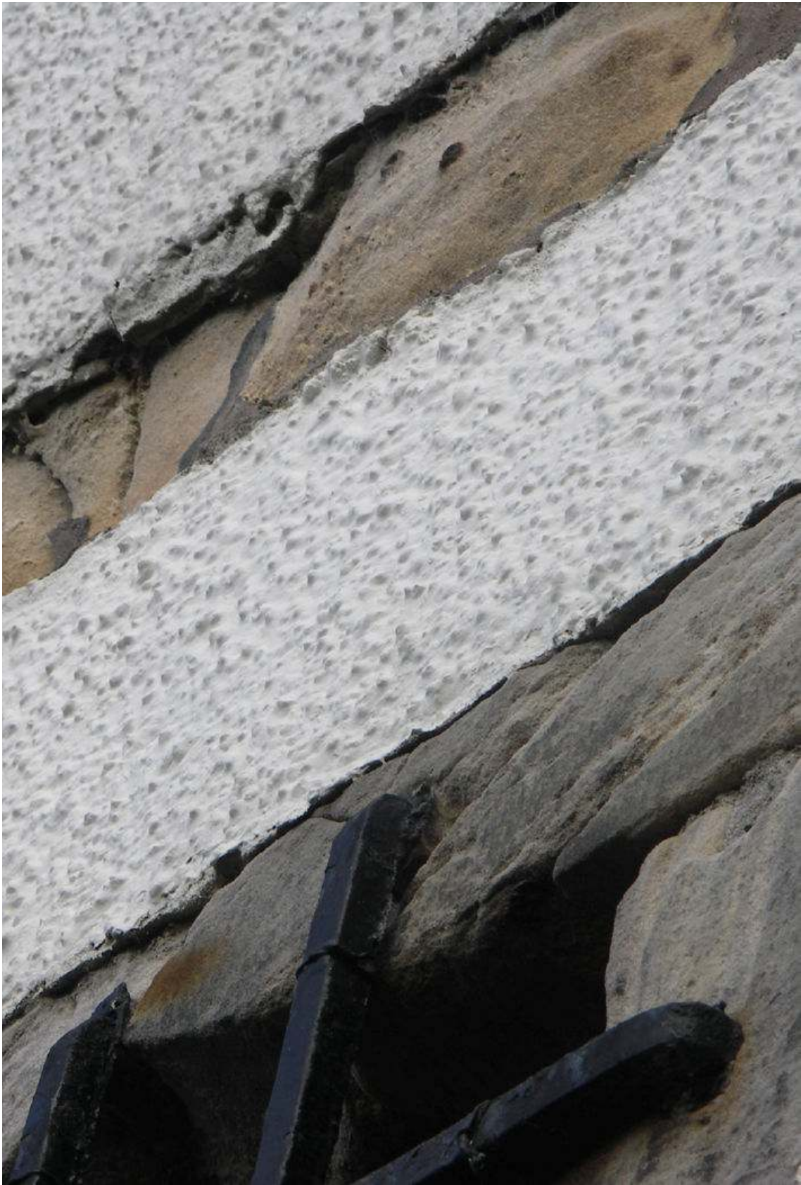
Fig 33: Detail of masonry decay accelerated by cement render.
